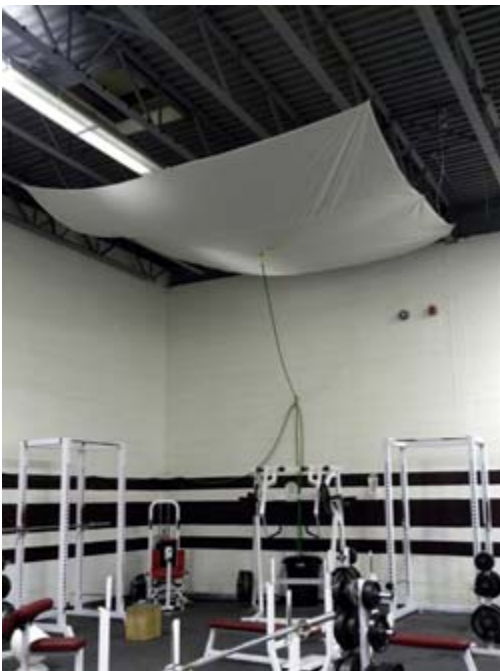
Serious roof leak in weight room, tarp was installed to catch the water and then is directed to a hose which empties into a garbage can sump pump system.
