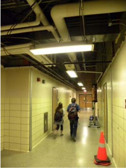
Wiring is open in ceiling waiting to be tied into the new wiring.
