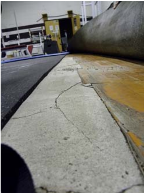
Attempts have been made to repair floor but the cement is now heaving.
