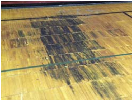
Continual water damage on the floor of the gymnasium
