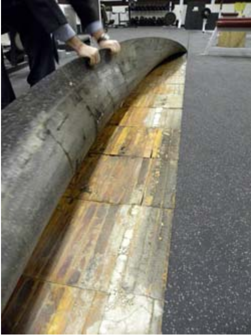
Serious floor heaves and water damage in weight room.
