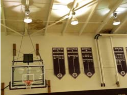
Several roof leaks in the gymnasium ceiling.
