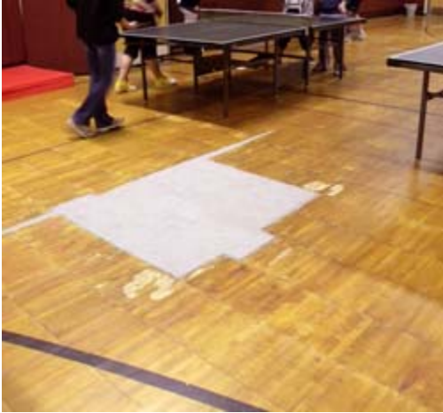
Floor in gymnasium had heaved and required repair - wood was cut and removed and replaced with cement. Floor is uneven in many areas.
